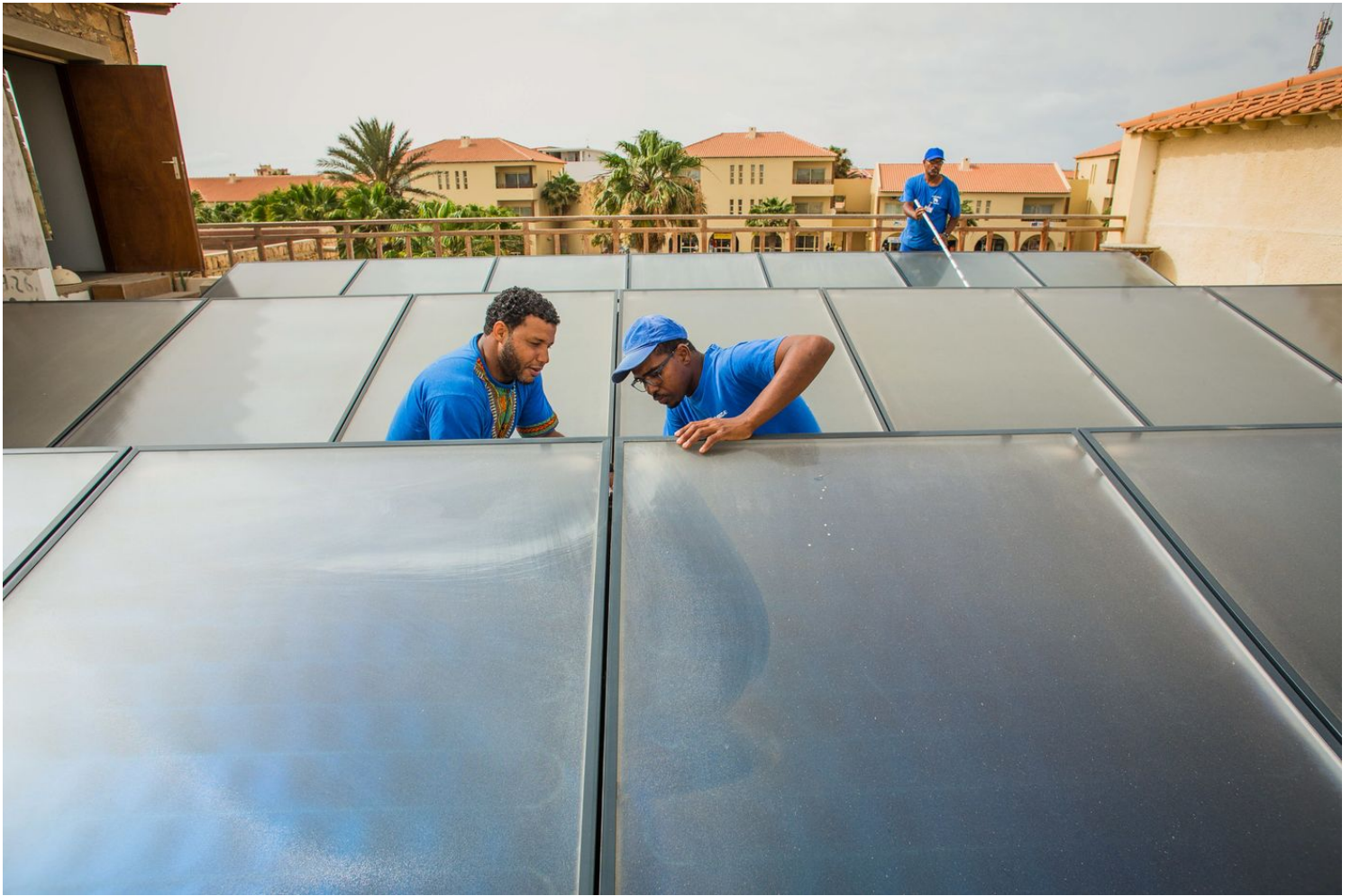
Solar panels being installed in West Africa's Cape Verde. Photographer: Chris Willan/The Travel Foundation
